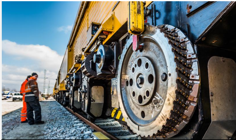
Rail milling train in operation. Image: „LINMAG Rail Milling Service“ on Linkedin © LINSINGER Maschinenbau GmbH
